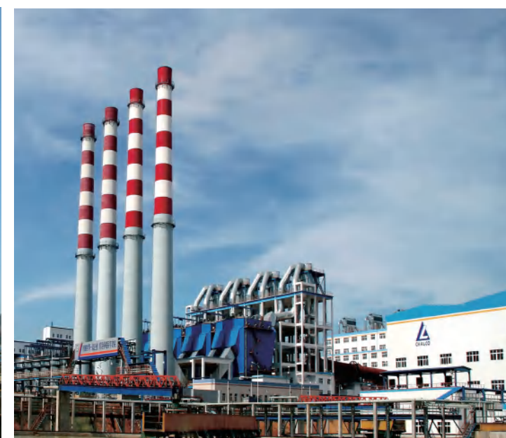
中铝中州铝业有限公司转窑及净化设备 Chinalco Zhongzhou Aluminum Co., LTD. Rotary kiln and purification equipment
