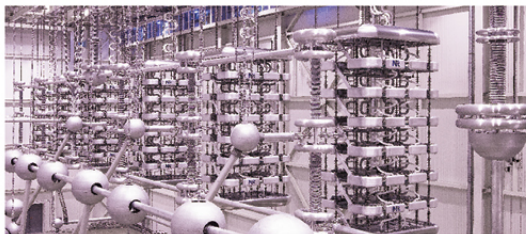
特高压晶闸管换流阀
